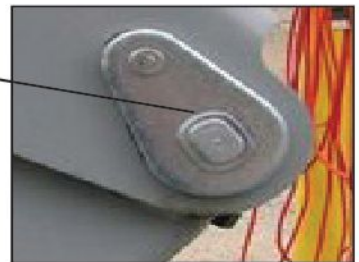
No rust. Pin has not rotated. Area is clean of dust/metal shavings
